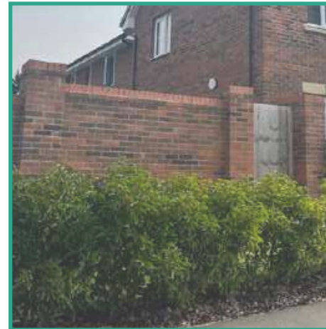
Red brick wall and wall posts with hedgerow to soften the wall's hard interface and rigidity
